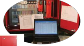
Elektrik Kontrol Paneli Electric Control Panel
